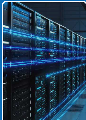
3. Data Center Hardware Deployment
