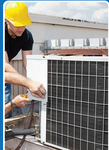
3. Air Conditioning Systems
