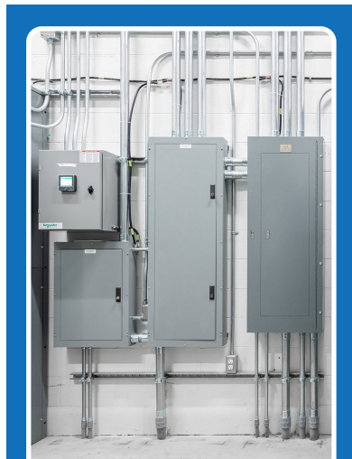
3. Power Distribution Solutions
